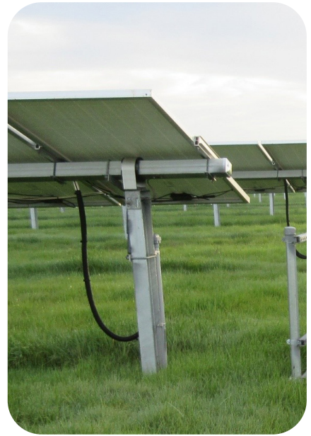
The tubing used on the wiring in this photo would seem to protect the wires from damage. The long, loose run actually encourages damage from lawn mowing equipment and the wind.
