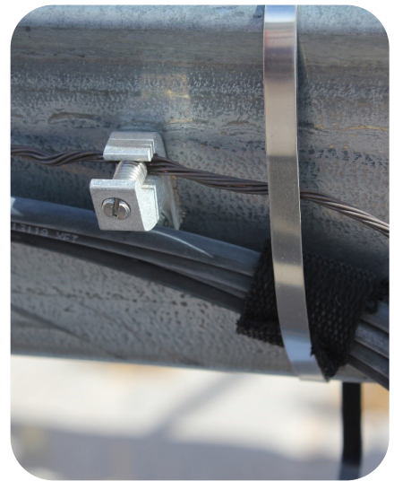
In the image above, effort was made to protect the cable jacket from potential abrasion from a metal cable tie. The risk is that this small piece of insulation may erode or slip and leave the cable jacket exposed to the metal tie at an unfortunate angle.
