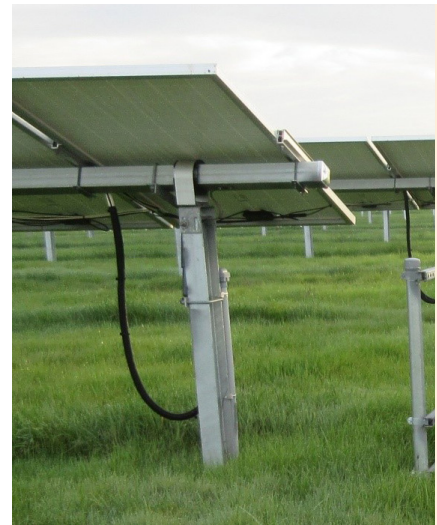
The tubing used on the wiring in this photo would seem to protect the wires from damage. The long, loose run actually encourages damage from lawn mowing equipment and the wind.
