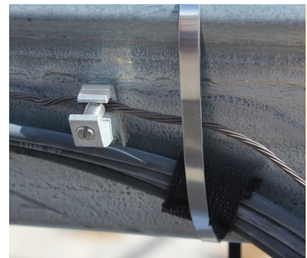
In the image above, effort was made to protect the cable jacket from potential abrasion from a metal cable tie. The fear is that this small piece of insulation may erode or slip and leave the cable jacket exposed to the metal tie at an unfortunate angle.
