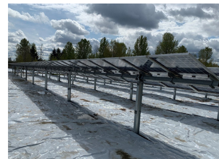
This project in Oregon utilizes a white ground covering to both increase UV radiation to the back of the modules as well to help mitigate growth of weeds and other ground coverings.
