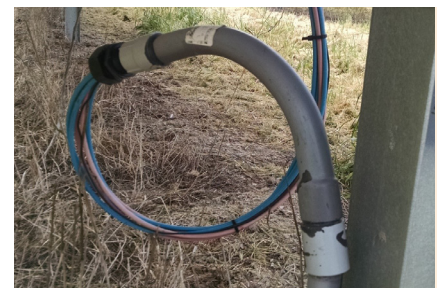
This conduit was damaged when the tracker went to the far east position every morning. The conduit also penetrated the module backing and cracked the glass.
