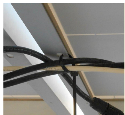
The nylon cable tie looped through the module hole is unlikely to last more than a year or two on a single-axis tracker application.
